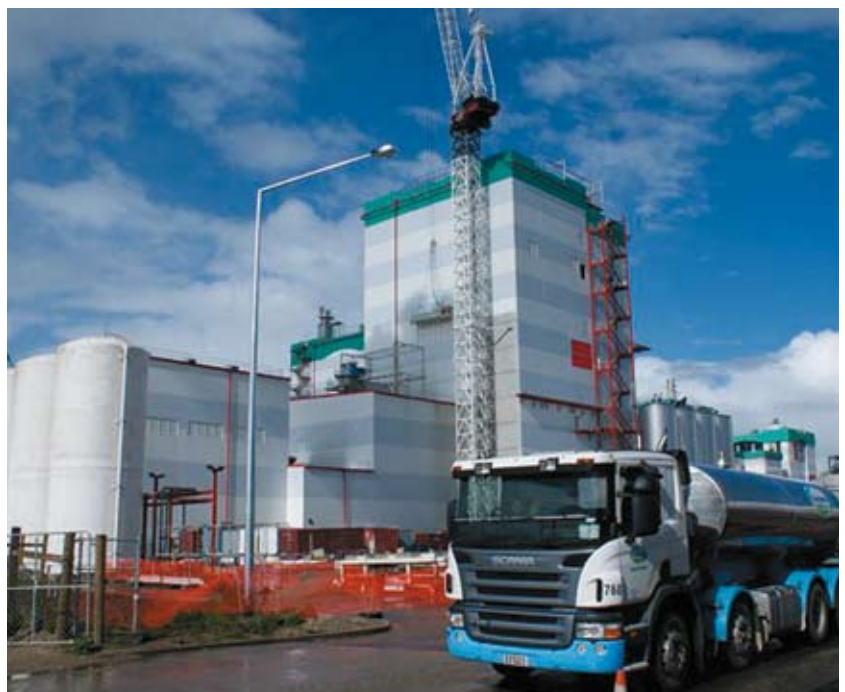
View of the Edendale site during construction of the ED4 Drier operation
